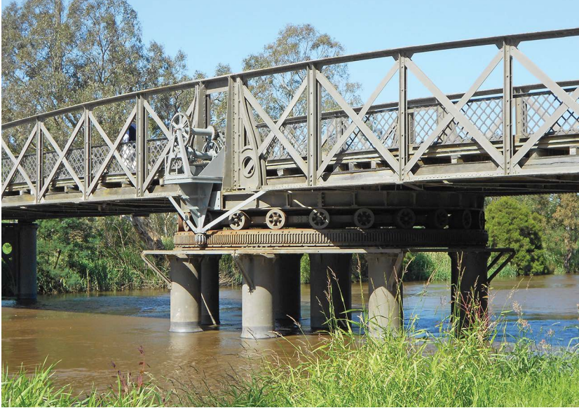
Figure 5.8: The Sale Swing Bridge, showing the central piers around which the deck pivots.
