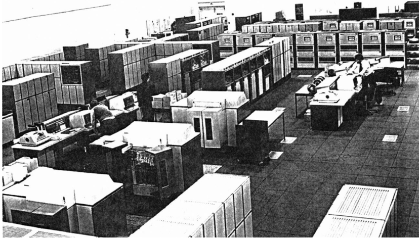
Figure 8.2: The PMSL computer room at Mixenden, Halifax. So much wonderful Sperry 1100 equipment.
