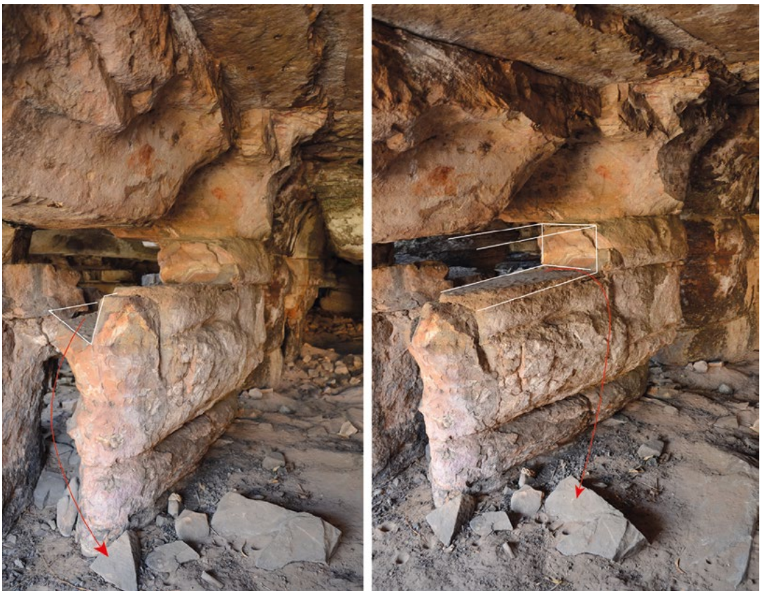
Figure 10.32 Partially removed pillar, with upper parts missing, southwestern sector.
