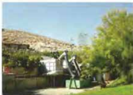
Figure 3: ROTAMAT® fine screens at lagoons in the Middle East
