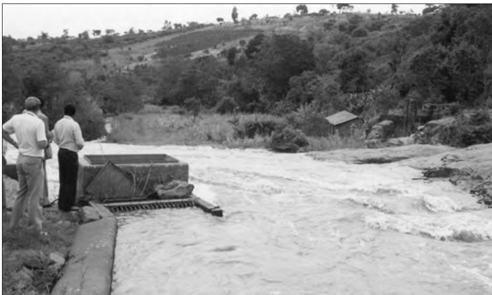
Figure 3.37: Intake weir washed away by the rains in 1983 693
