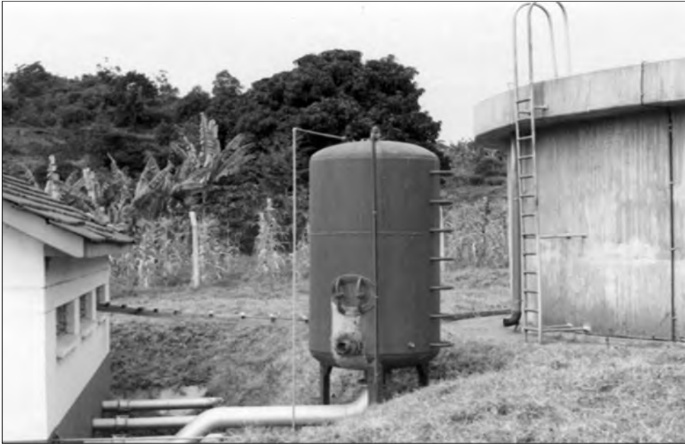
Figure 3.38: A Surge vessel (not working for fourteen months due the breaking down of the compressor 1983 695 .
