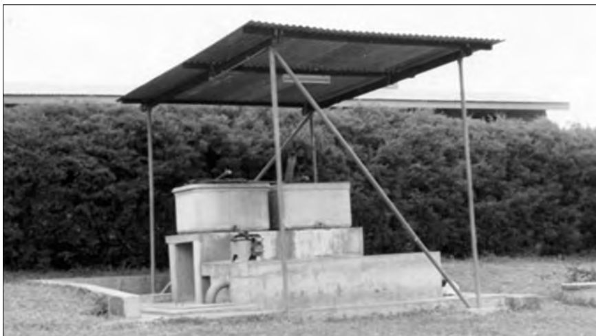
Figure 3.19: Mixing chamber in Rongo 317
