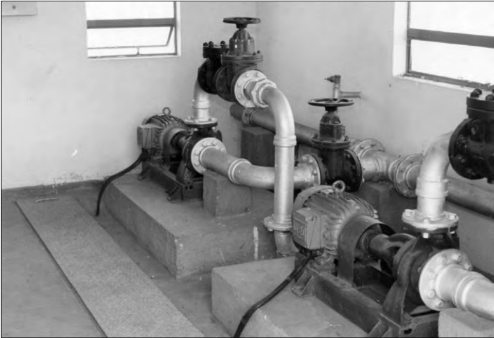
Figure 3.17: High lift pump worked satisfactorily although poorly installed by 1983 311
