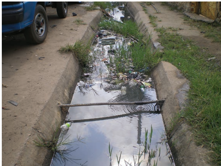
Photo 17 The drainage channel is blocked as it is not cleaned regularly.
