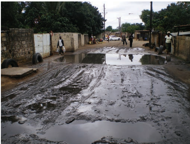
Photo 12 Movement of vehicles on the unsurfaced roads creates undulations and depressions, where the water collects and stagnates.
