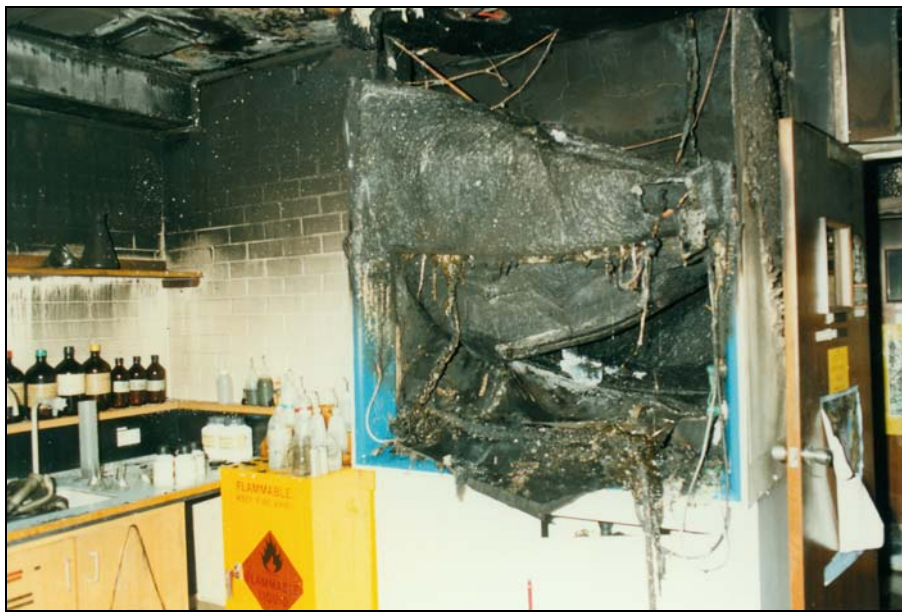
Damage to the Lab wing after the February 1996 fire
