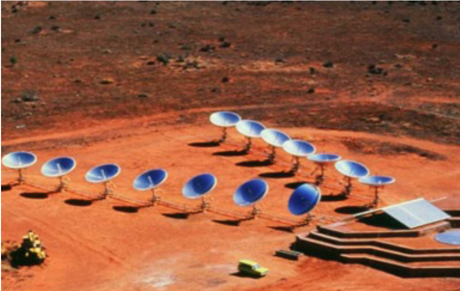
1. White Cliffs solar thermal power station, aerial view
