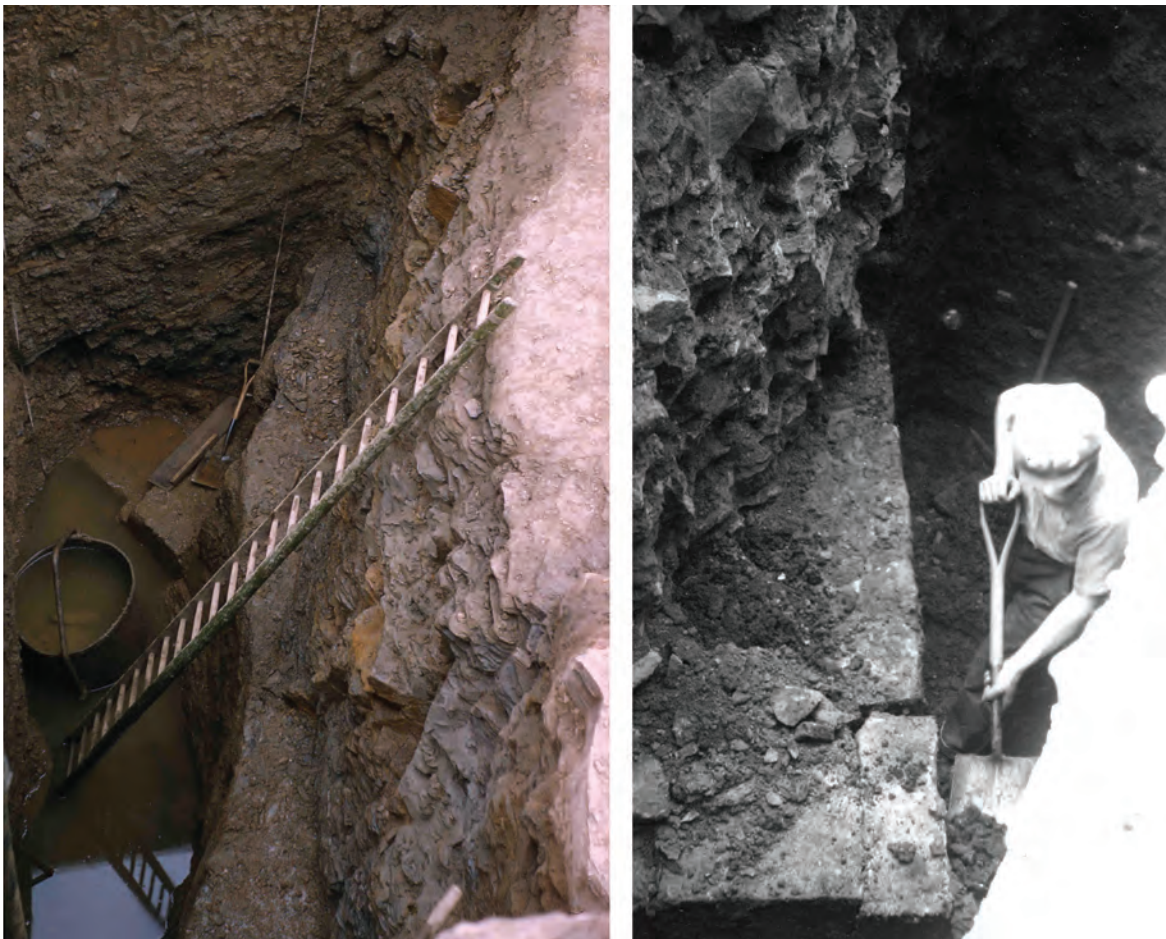
Figure 4.10: Photographs of foundation shafts taken on site in the late 1950s. The Butcher archive contains a wide array of both colour and black and white photographs, taken by Cyril James, Ray Newton and Leslie Butcher. Courtesy of Museums Sheffield.
