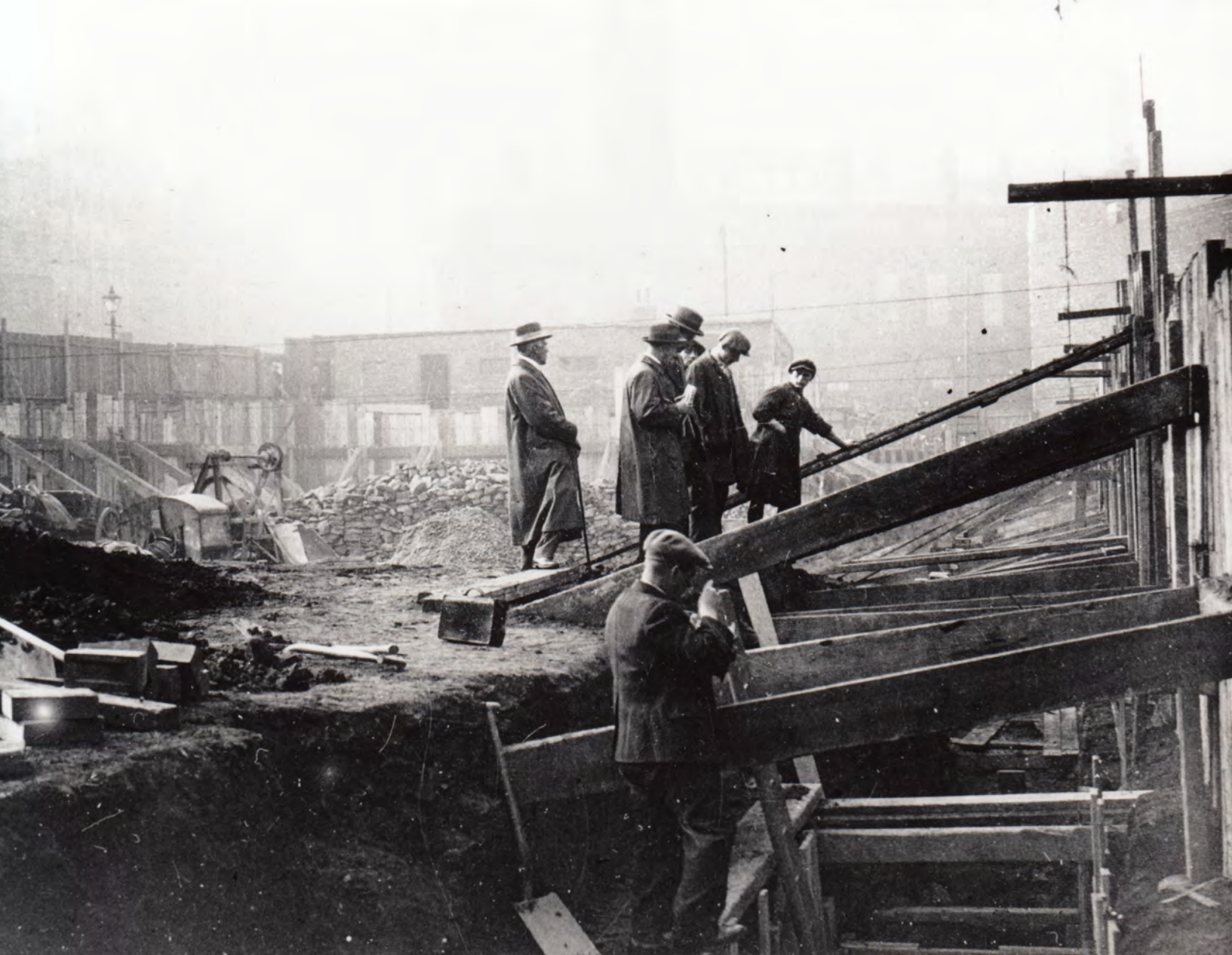
Figure 2.3: A photograph taken by Joseph Himsworth when he visited the building work on Castle Hill in October 1927. He was accompanied by Leslie Armstrong and J. R. Wigfull. A similar photograph also taken at this time is included in Himsworth's diary. Armstrong is second from the left in the group in the middle of the picture. Courtesy of Museums Sheffield.
