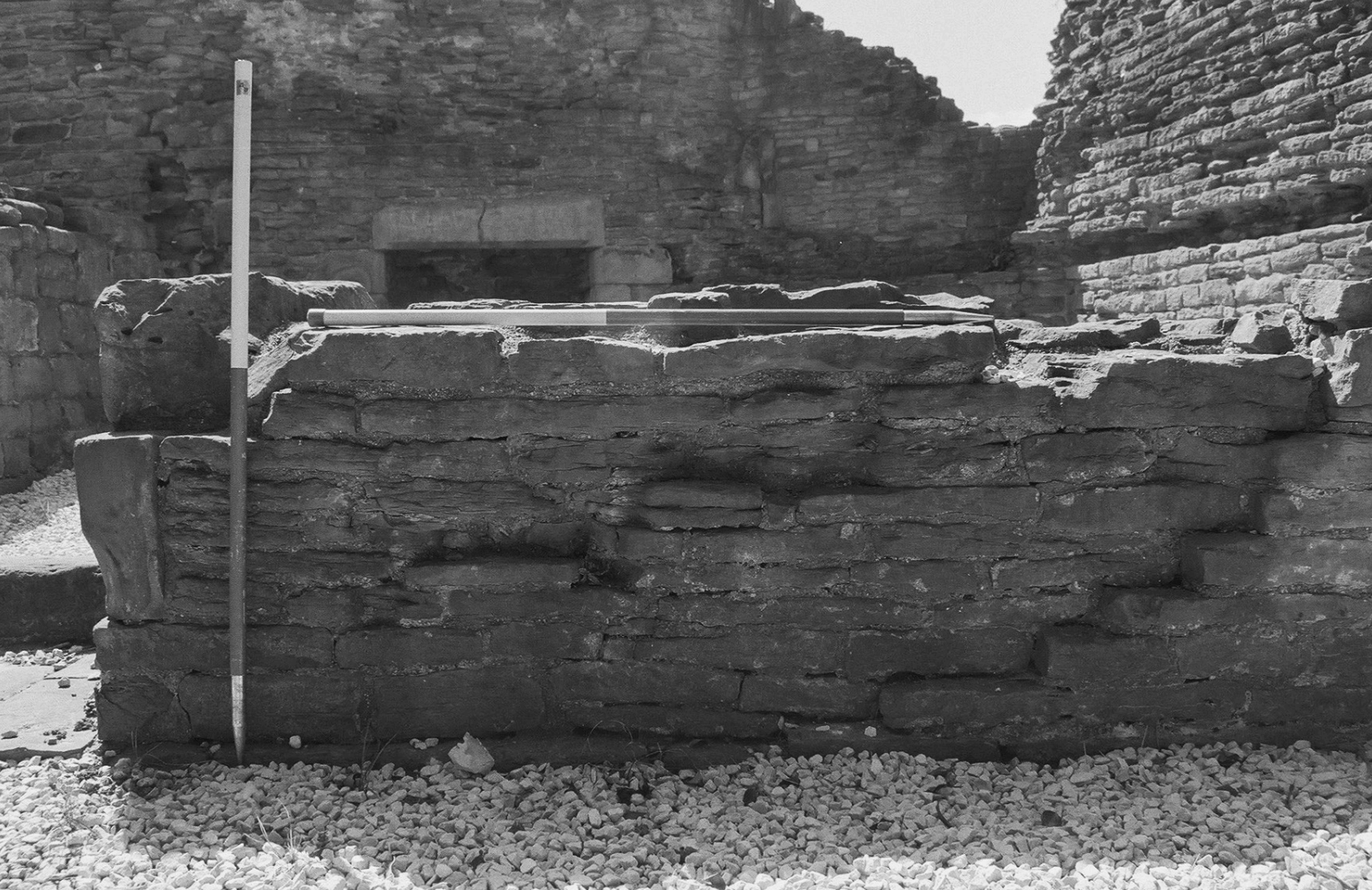
Figure 8.15: The three-storey tower at the north end of the long gallery. Scars on the west wall reveal the former presence of a staircase. At the rear of the photograph is the top of the fireplace in the west wall of the two-storey tower. Wessex Archaeology.
