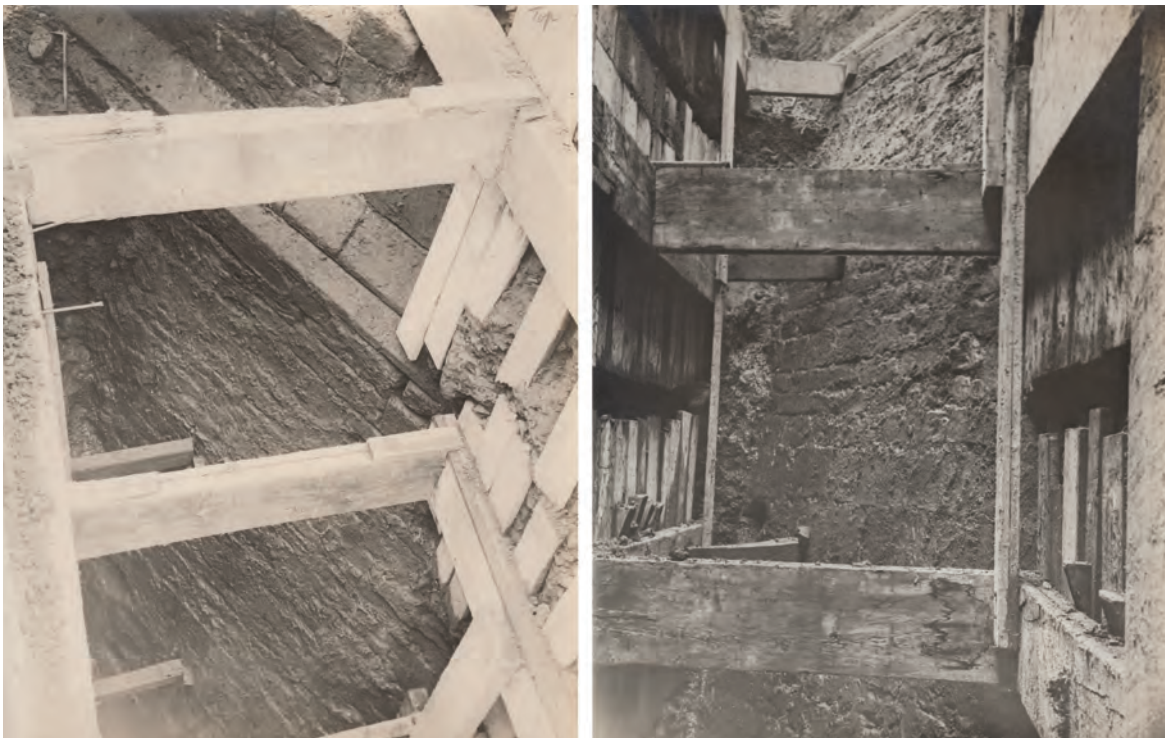
Figure 3.11: The lower walls of the gatehouse projecting into the moat. Signs of cannonball impact can be seen at the lower left of the right-hand image. Courtesy of Museums Sheffield.
