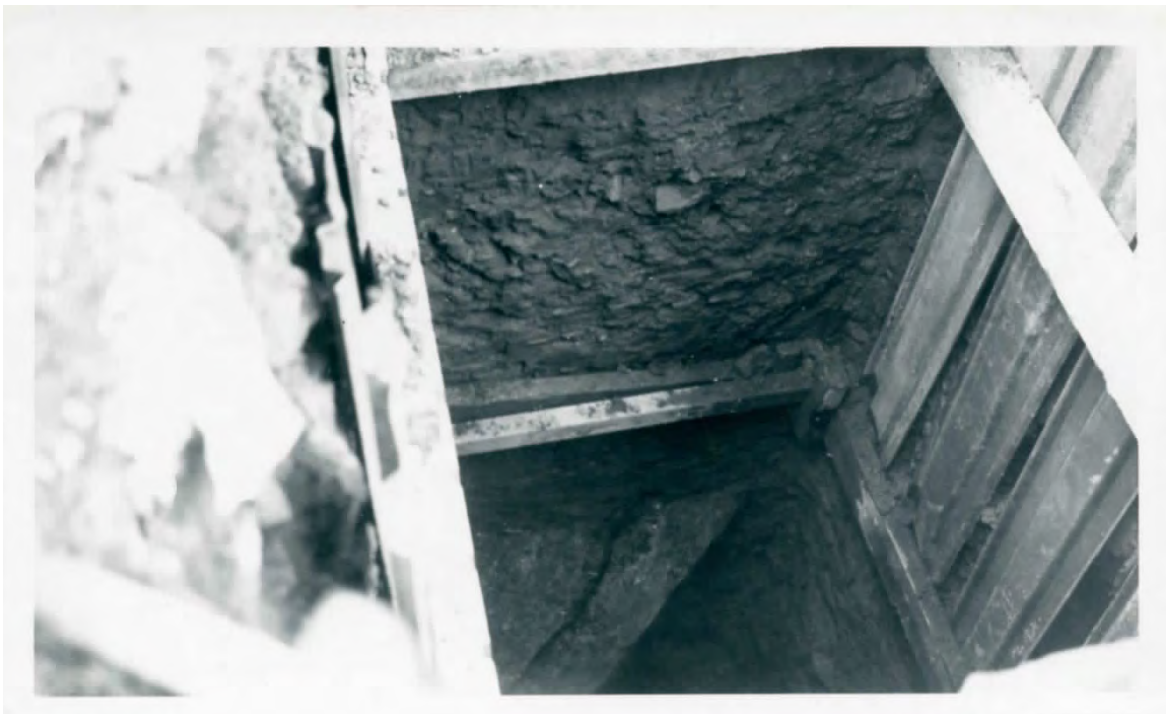
Figure 5.3: Looking down foundation shaft E19 from the north-east. This photograph shows the use of shuttering by the construction workers. Courtesy of Museums Sheffield.
