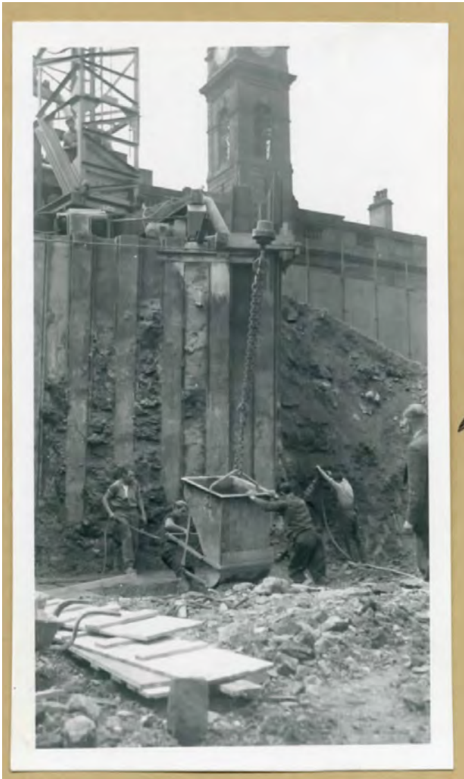
Figure 4.8: Workmen filling a bucket – or kibble as it was known in mining parlance – during construction work on Exchange Street. Courtesy of Museums Sheffield.
