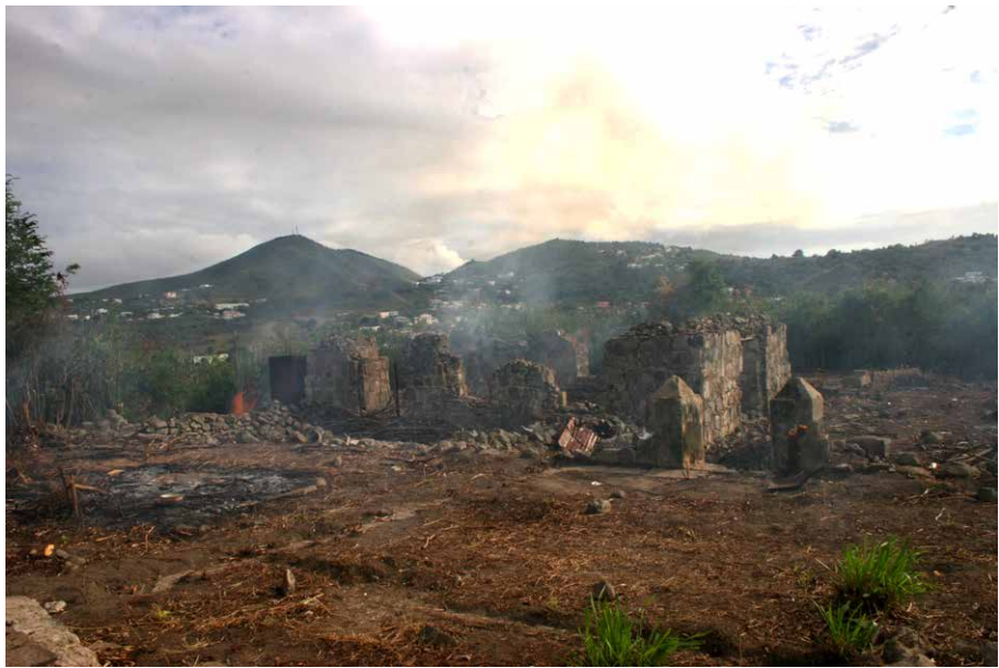
Figure 12.4: View of the foundations of the estate house (in front) and the curing house during the clearing of the site.
