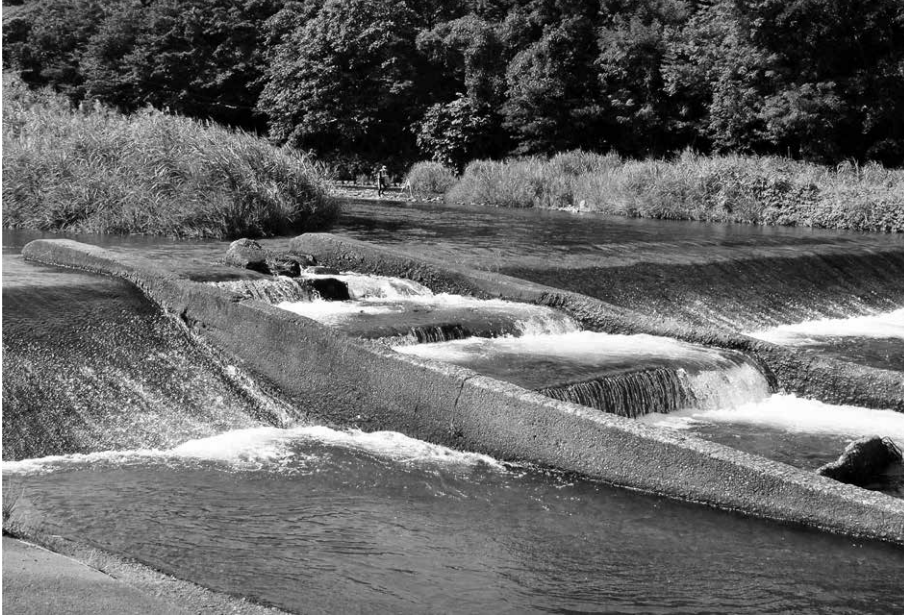
Figure 6. The current state of the diversion weir No. 5 in Fig. 4. Photograph by Ishii, A., August 2014.
