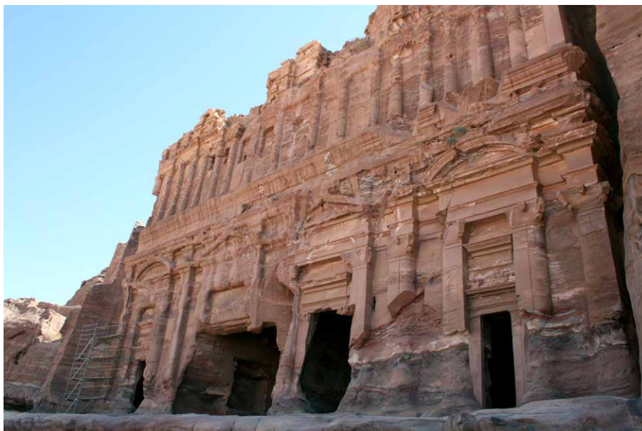
Figure 9. Note patterns of sandstone deterioration at Petra tombs: water acts to deteriorate sandstone in several ways. One way that this occurs is when salt laden water is absorbed by sandstone at the base of tombs, producing characteristic keyhole shape for ground level doors, also sandstone spalls away from facades, taking with it tomb embellishments. photo by Diego Delso, Wikimedia Commons, License CC-BY-SA 3.0
