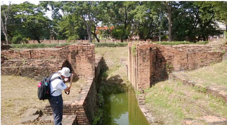
Figure 9. At the World Heritage Site of Ayutthaya, many canals have fallen into disuse thereby restricting the water drainage capacity in the event of heavy rainfall.
