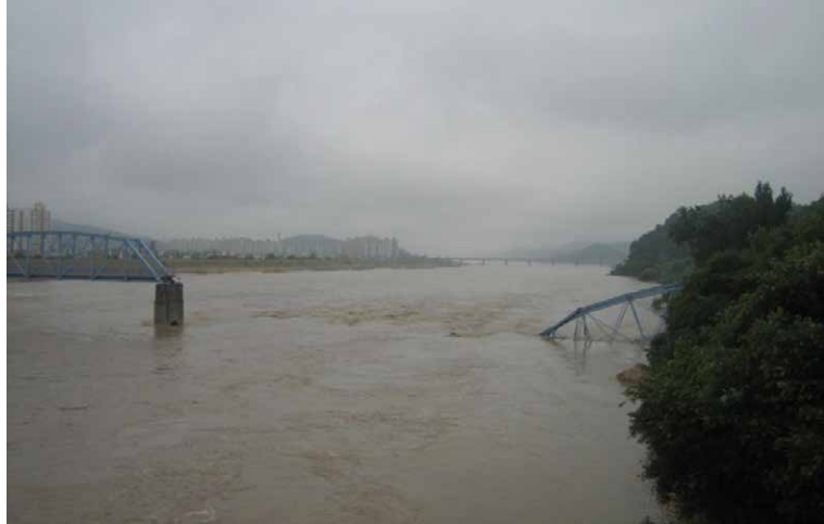
Figure 9. The destroyed Waegwan Bridge (CHA 2013).
