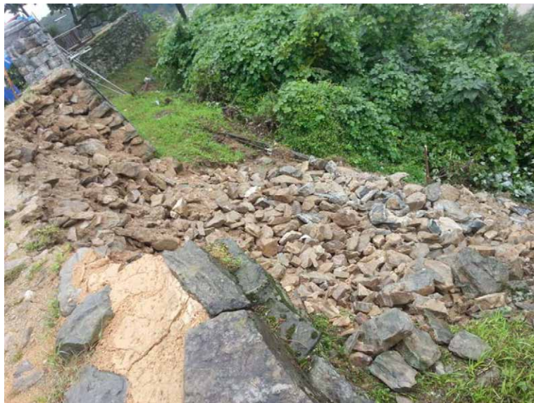
Figure 10. The collapsed section of the Gongsanseong Fortress (CHA 2014).
