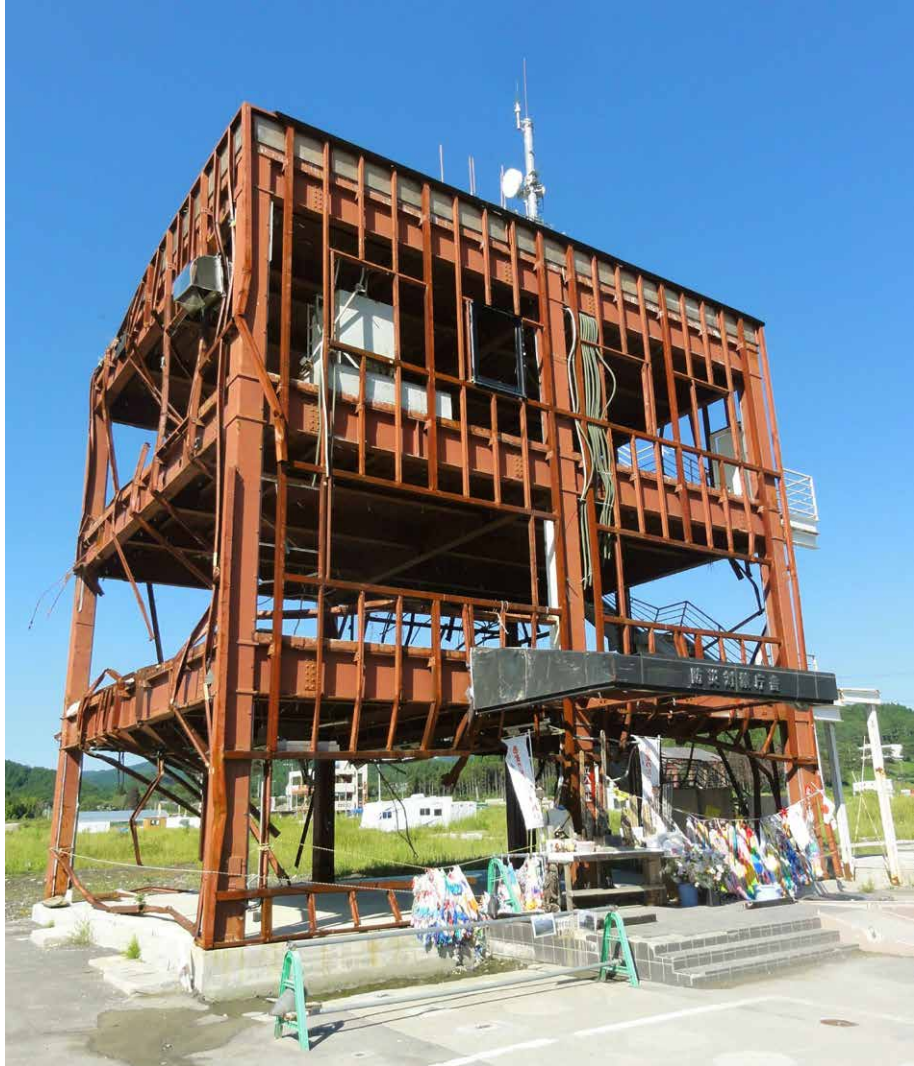
Figure 4. The Disaster Mitigation Office of Minami-sanriku town, Miyagi Prefecture, on the 7 th of September 2012.
