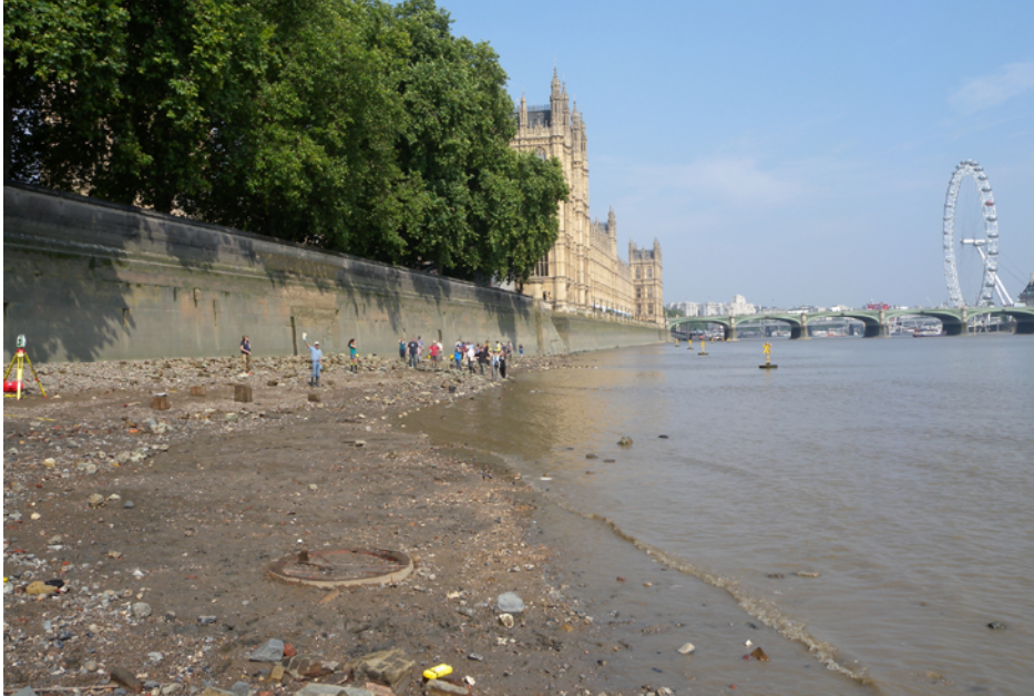
Figure 14.3 Recording WWII bomb damage to the river wall upstream from the Palace of Westminster, London. (Photograph by N. Cohen. Copyright reserved)
