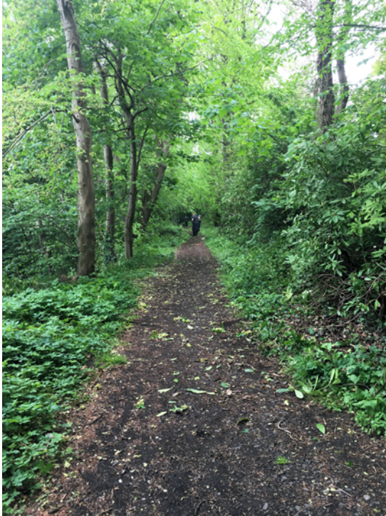
Figure 16.2 The trail emerging as we clear vegetation from the path. (Photograph by Paul Murtagh. Copyright reserved)
