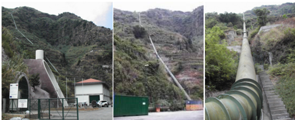
Figure 2. Socorridos pumping station – outside view (on the left). Socorridos-St. Quitéria steel pipe (on the centre and on the right)
