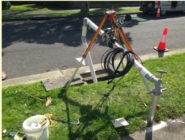
Figure 7.11 Experimental set-up to check discharge measurement devices. Source: Peter Poelsma (University of Melbourne).
