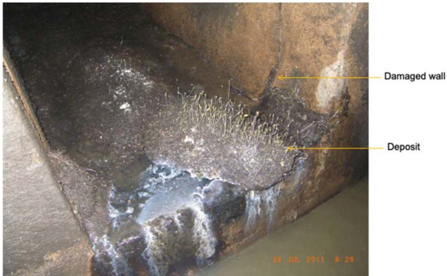
Figure 3.3 A sewer section where sediment deposit and damaged wall hinder installation of sensors for discharge measurement. Source: Université Gustave Eiffel.
