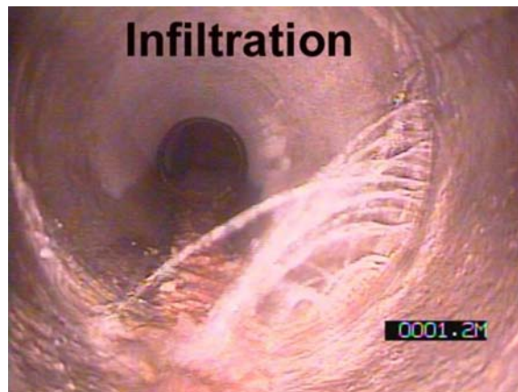
Figure 3.47 Clear example of infiltration of groundwater into a sewer pipe. Source: Deltares.
