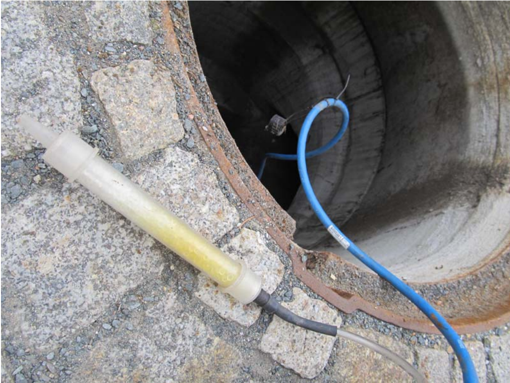
Figure 7.20 Half-used silica capsule of a water level sensor. Source: Jakob Benisch (TU Dresden).
