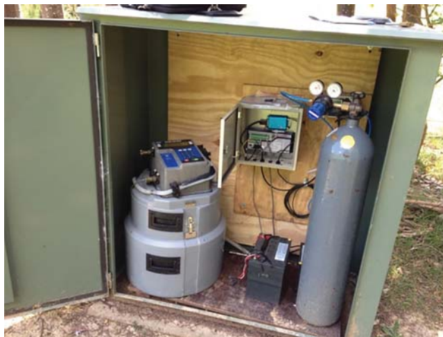
Figure 7.7 Metal cabinet housing monitoring devices. Source: Peter Poelsma (University of Melbourne).
