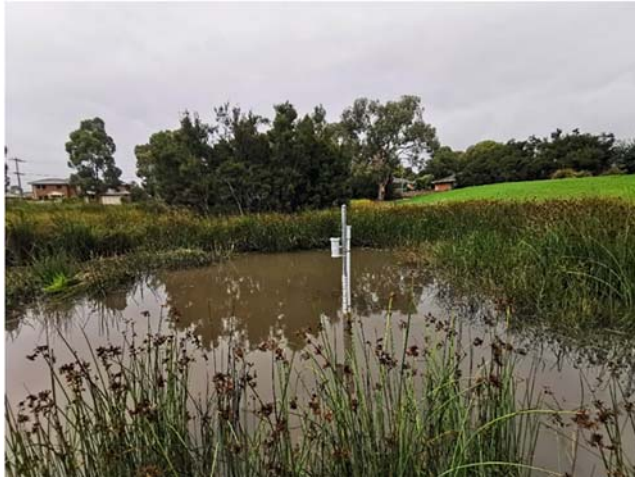
Figure 7.8 Ultrasonic (left) and capacitive (right) sensors for water level monitoring installed in PVC pipes and above the water to avoid any vandalism – wetland in Melbourne, Australia. Source: Frédéric Cherqui (INSA Lyon).
