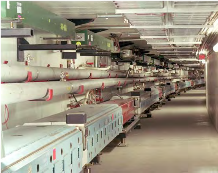
Fig. 5. The Recycler (top) and the Main Injector (bottom) rings installed in a common tunnel.
