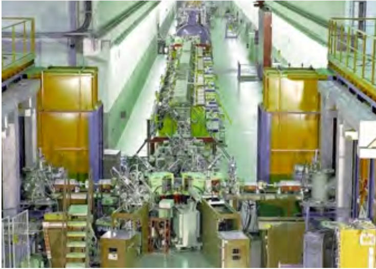
Fig. 2. View onto the Unilac during the installation phase with the two Faraday cages for the ion source platforms (left and right), the beam transport lines to the RF-linac, where charge and isotope separations are performed, and the Wideröe-type pre-stripper accelerator (yellow) in the foreground. The Alvarez-type post-stripper accelerator (violet) is visible in the background. The stripper and the following charge analyzing system are installed in between. (All photographs in this chapter are by Zschau, GSI)
