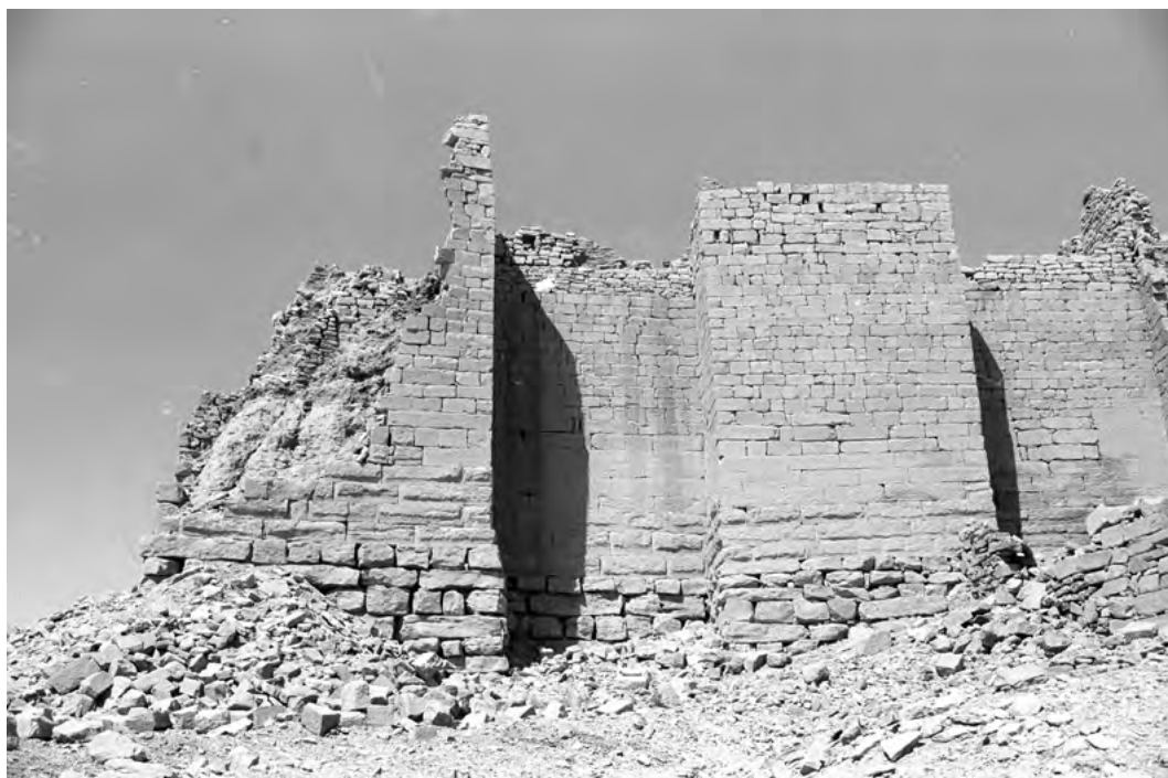
Figure 17. The foundations of bastions T36 and T37 of the city wall, from the south. (A. Solazzi 1986 © MAIRY)
