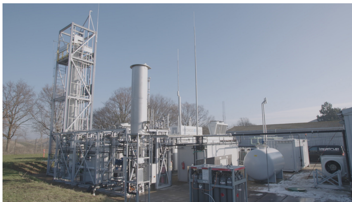
Figure 6.6 Picture of a 1-MW power-to-methane system at a wastewater treatment plant. The stirred bioreactor with bubble formation in a column is on the left. This picture was taken at Electrochaea's patented BioCat plant in Avedøre, Denmark, which is a demonstration-scale system to store biogas as renewable natural gas in the Danish natural gas grid.
