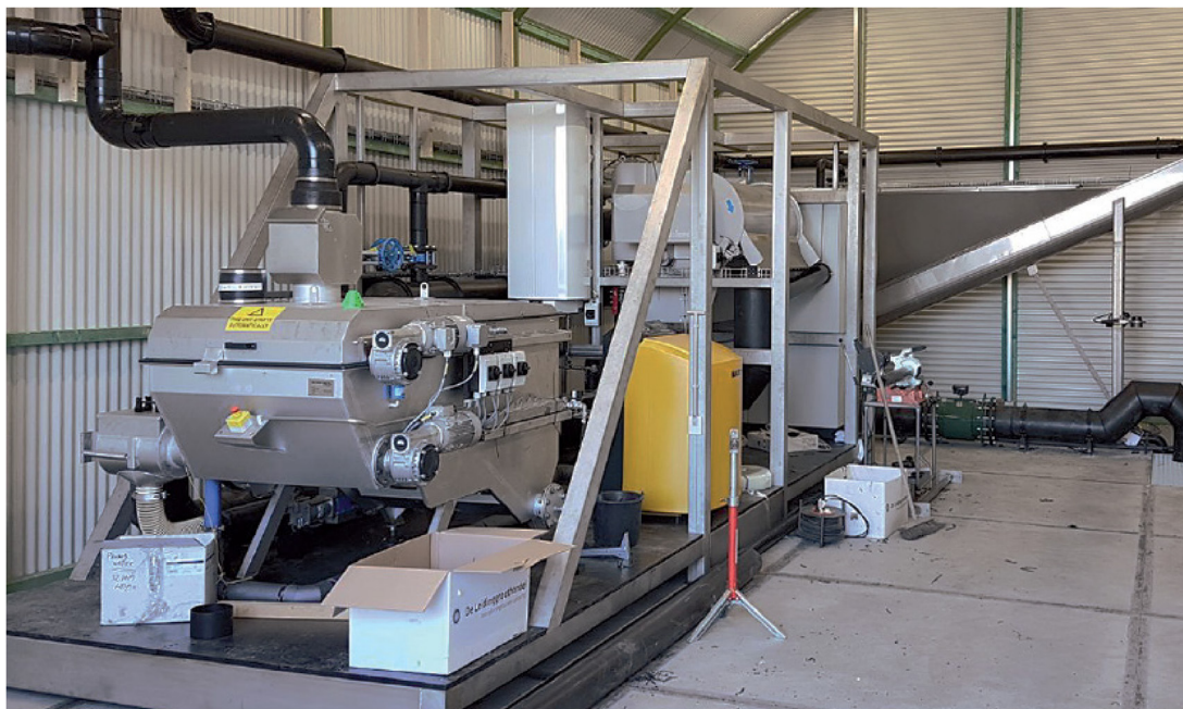
Figure 8.3 An RBF system is demonstrated at the sewage treatment plant of Geestmerambacht (The Netherlands).
