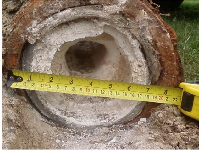
Figure 10.3 Unwanted inorganic scale within water pipework.
