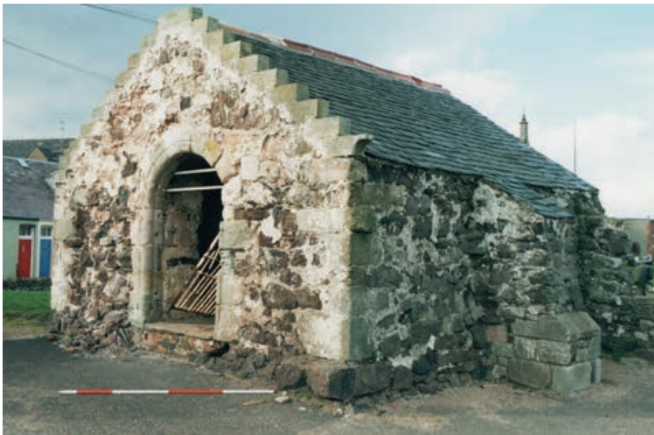
Fig. 4.32: View of the south porch from the SE taken in 2000, before commencement of repair works
