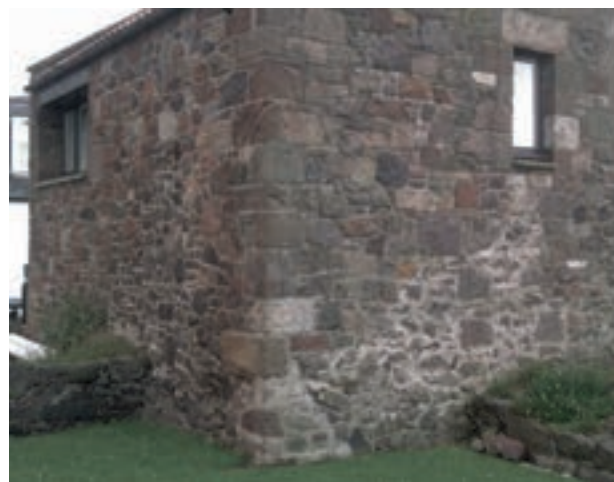
Fig. 4.42: The south and east walls of Church Cottage contain reused stonework from the church
