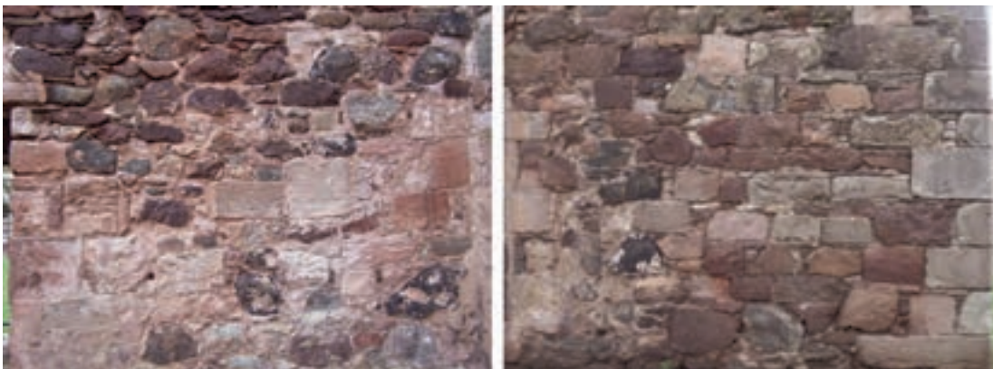
Fig. 4.39: Much of the general lower walling of the 17th century church, contains reused stonework, this demonstrably from the Old Kirk
