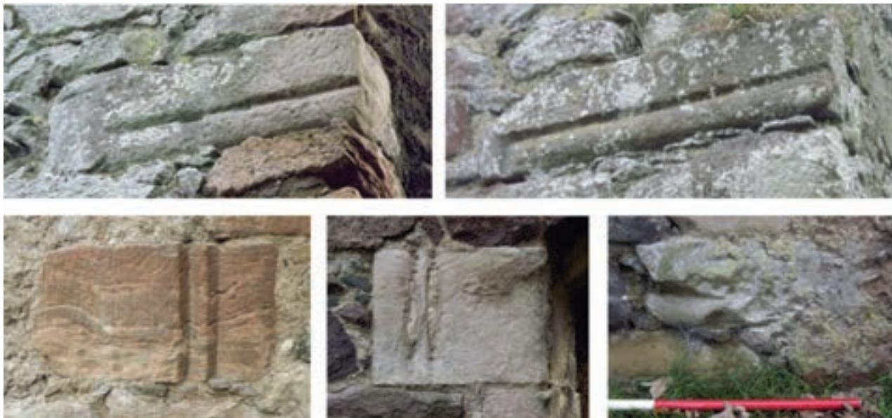
Fig. 4.40: Individual stones displaying moulded detail: lintels with quirked rolls (above), and jamb stones with twice-quirked angle rolls, and part of a pier base, inverted (lower right)
