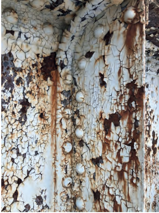
Figure 2: A nineteenth-century railway bridge at Björneborg, Sweden. How can we take care of this heritage when the nature of the authentic painting materials has changed and few painters have the appropriate skills to use linseed oil paints? This issue requires communication about the interaction of tangible and intangible elements of materials and working procedures. Photograph by Sven-Olof Ahlberg.
