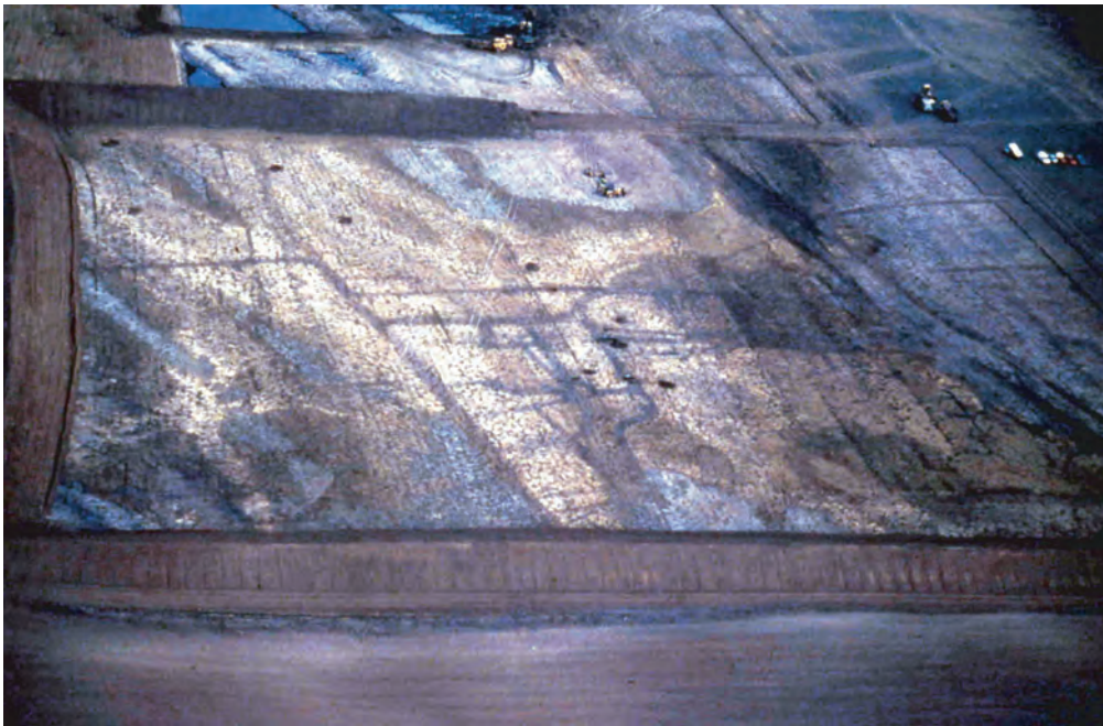
Fig. 12 Aerial photograph of Lydd 1 after topsoil stripping (from west, looking east) (photo taken by the late Graham Alleyne). (© UCLFAU)
