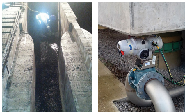
Figure 2.2 A large flume influenced by poor maintenance procedures allowing grit build up
