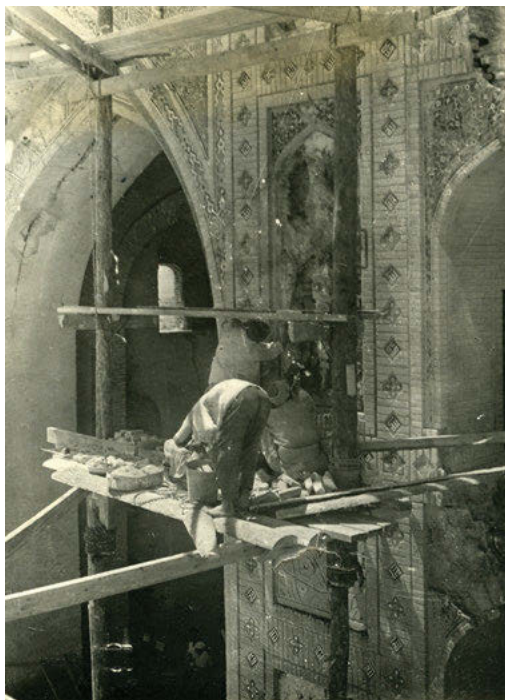
Figure 11.24: “Work on reinforcing the structure on the right-hand side of the mosque’s door, Anau, 1936”. Photo by Nikolai Mikhailovich Bachinskii. Archive of the Institute for the History of Material Culture, Russian Academy of Sciences.
