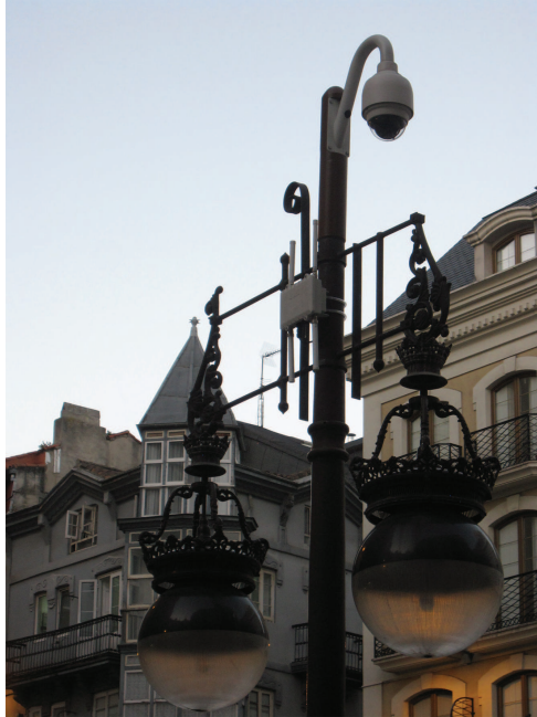
Figure 8.16 Street light in Santander.
