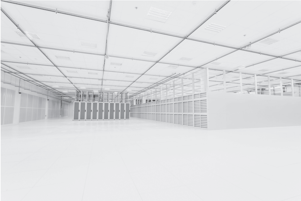
Figure 15.1 One of the server rooms in GigaTech’s East London facility Source: https://jamesbridle.com/works/the-cloud-is-a-lie . Photo by author.
