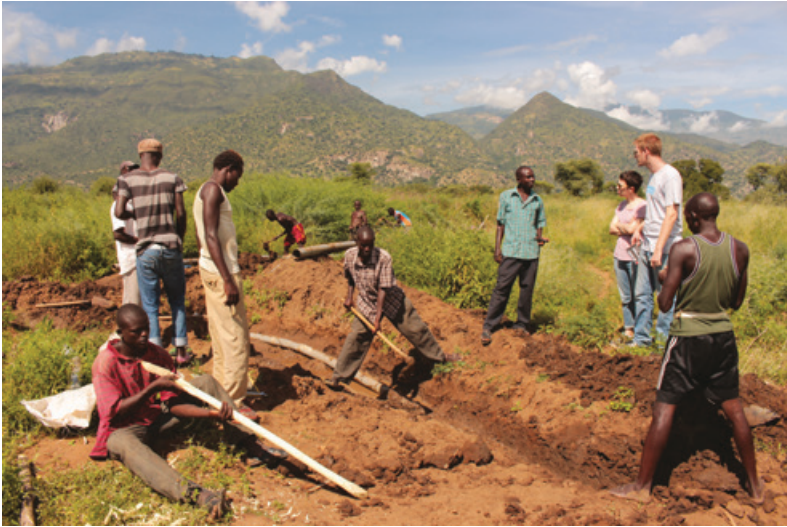
Figure 8.2 Noah Kiplagat, PROCOL Kenya citizen scientist, helps to dig a trench for the piping of the irrigation scheme.
