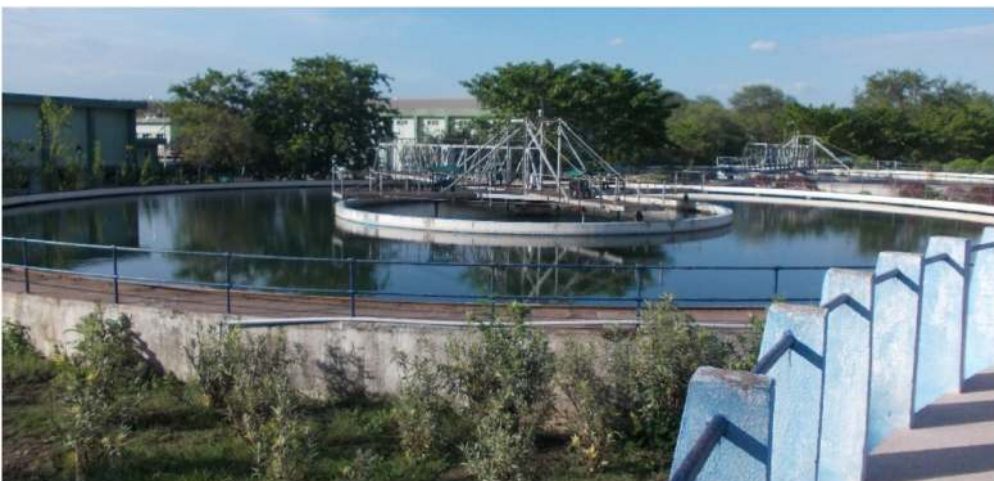
Figure 2.9 Flocculation chamber in water treatment plant (courtesy of Nagpur Municipal Corporation and Orange City Water Private Limited, Nagpur, India).
