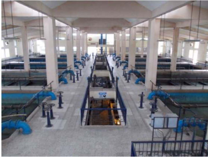
Figure 2.11 Filter house in water treatment plant (courtesy of Nagpur Municipal Corporation and Orange City Water Private Limited).
