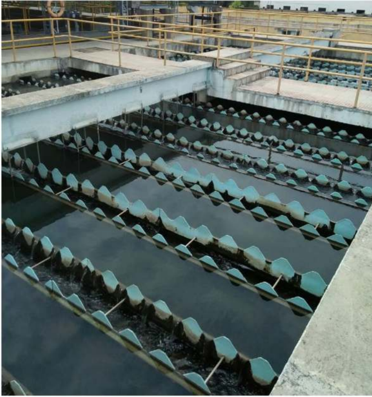
Figure 2.7 Pre-sedimentation tank in a water treatment plant (courtesy of Nagpur Municipal Corporation and Orange City Water Private Limited, Nagpur, India).
