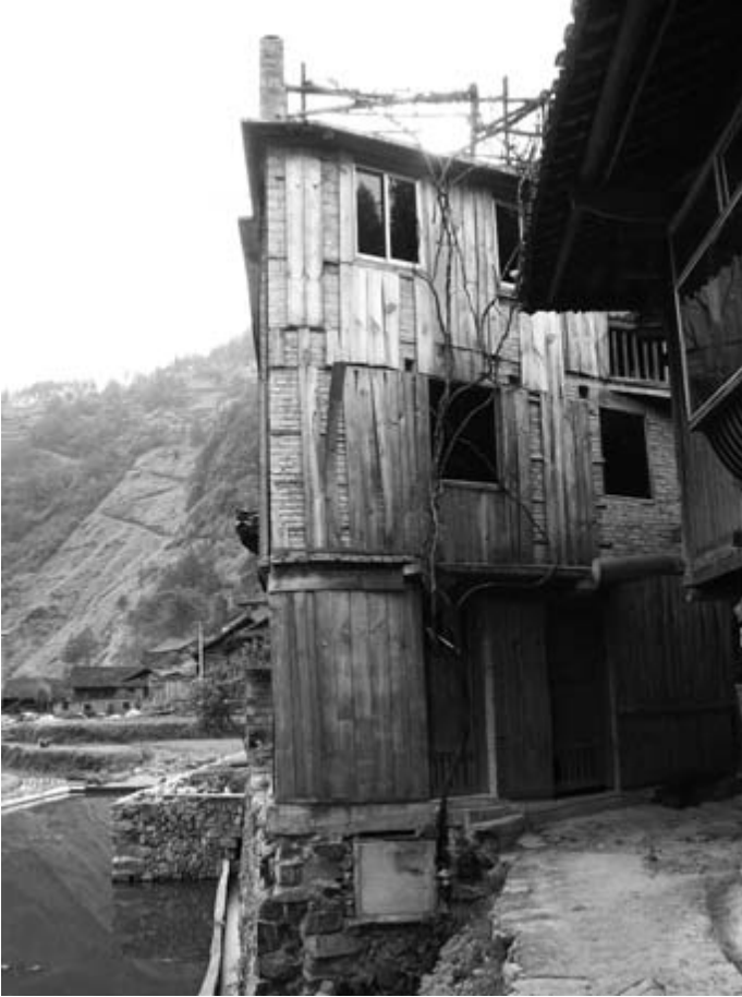
FIGURE 4.3. Wooden planks were used to cover up brick and concrete walls in Upper Jidao, but over time they warped and fell off (2006). Photo by the author.
