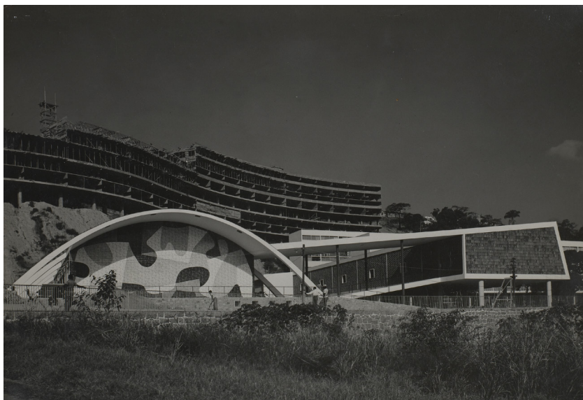
Figure 5.1: Affonso Eduardo Reidy, Pedregulho housing block under construction (Rio de Janeiro). As is clear from this picture, the community program was concluded before the residential block, revealing the prominence of the “common space” in the definition of the new community. Source: Brazilian National Archives
