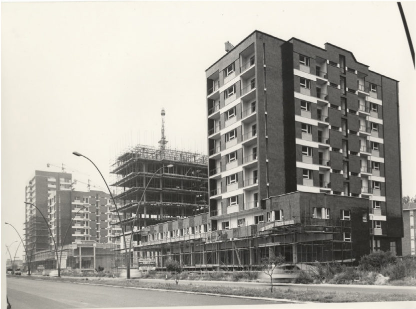
Figure 6.7: The construction site of the first four towers built along Corso Roma by the insurance company INA Assicurazioni and the small building company Deambrosi & Franchino in the late 1960s. Courtesy of the Archivio storico INA Assitalia
