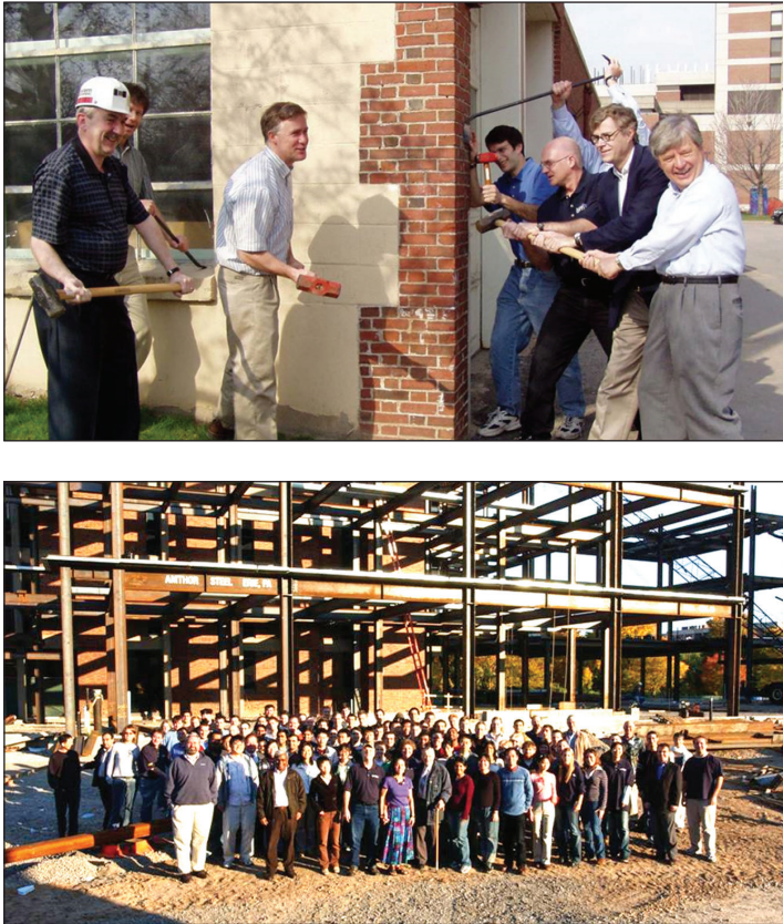
Figure 3.2. (top) Optics faculty members start the demolition of the old machine shop building; (bottom) Optics faculty, students, and staff pose during a brief pause in construction.
