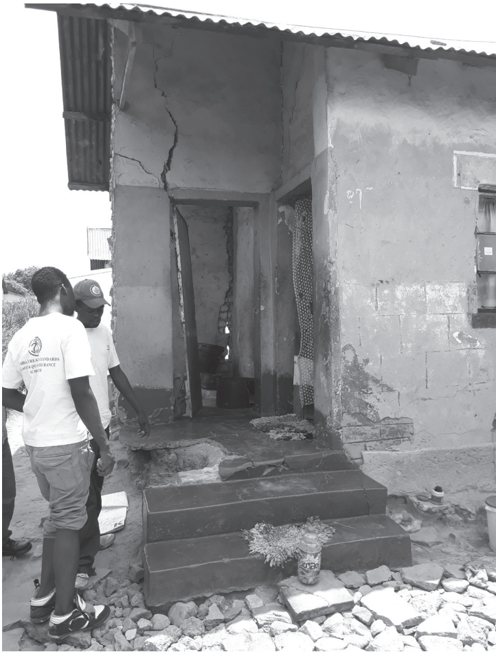
Figure 9.4 Cracked houses in Mufulira. Photograph by the author.
