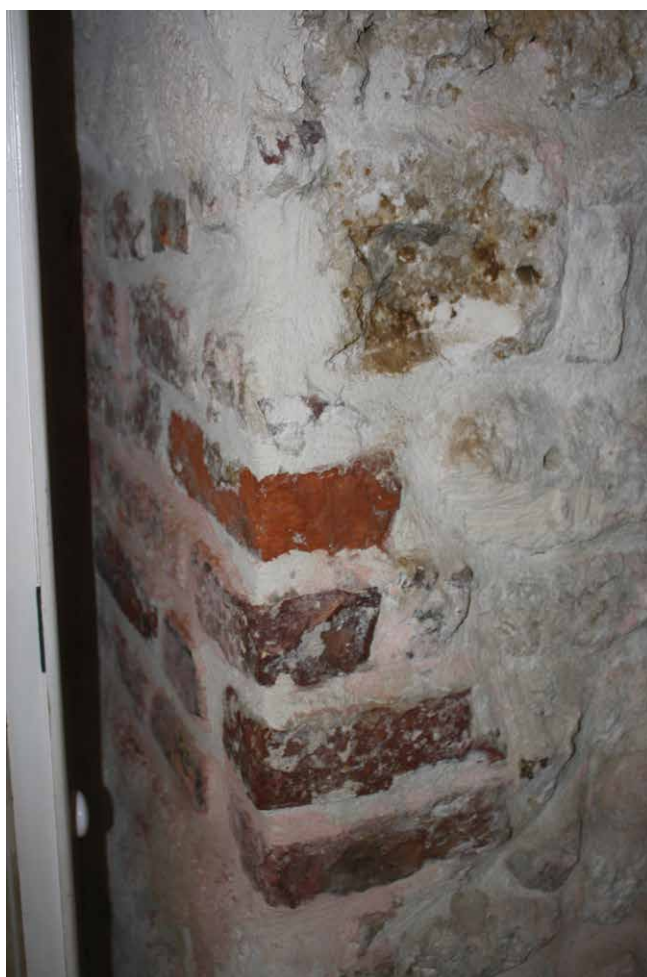
Figure 20.2. Former ballast incorporated into the building fabric at Arlington House Museum, Speightstown (Niall Finneran).
