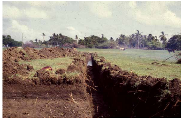
Figure 2.2. View of the Heywoods site (looking east) during the 1995 project showing the 2 m deep trench dug by backhoe to expose stratigraphy (Scott Fitzpatrick).
