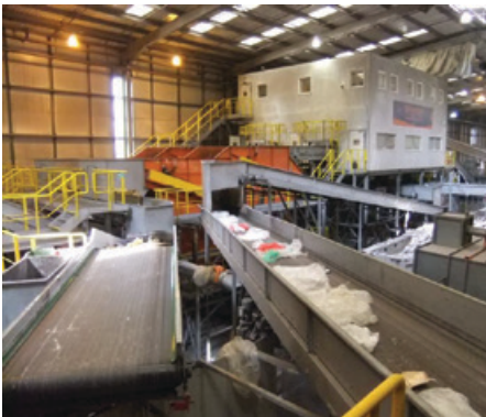
Material recovery facility for sorting mixed recyclables, London, United Kingdom (Urban Greendom).
