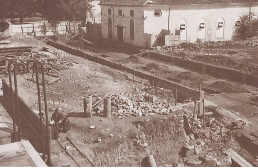
FIGURE 11 The old factory building at the back and the construction site at the front, 1934 COURTESY OF EMRE ÖNCÜ
