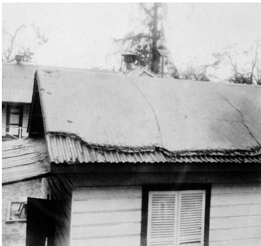
Figure 4.8. Two ash layers exposed on a roof in Rabaul.
