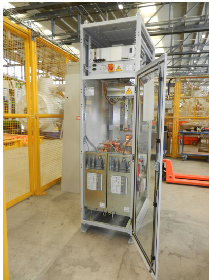
Fig. 1. In-vacuum switch based 2 kA energy extraction system.
