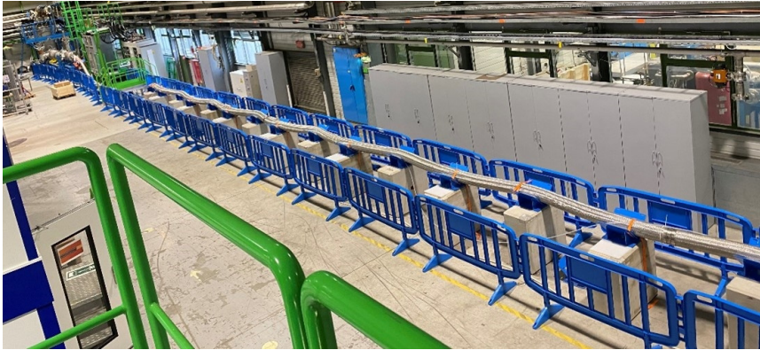
Fig. 4. View of a demonstration Cold Powering System – Demo 2 – tested at CERN for cryogenic and electrical qualification. The SC Link is 62.5 m long and it contains a full cross section \text{MgB}_2 cable assembly of the type needed for the powering of the HL-LHC Triplets.
