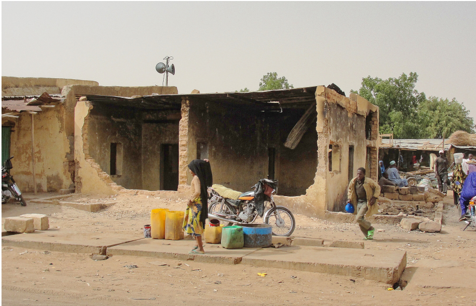
Figure 4.3: Burned-down police station at the main market. Photo: Jannik Schritt.
