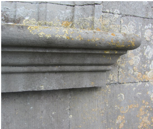
Figure 7.4: Details of the dressing of the stonework on the garden front of Castletown House, County Kildare, showing a window sill.
