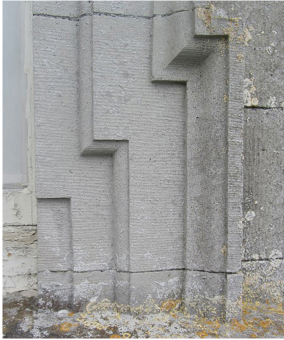
Figure 7.3: Details of the dressing of the stonework on the garden front of Castletown House, County Kildare, showing the base of the lugged architrave.
