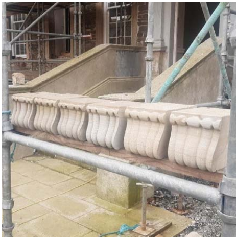
Figure 6.19: New carved keystones on display for 30 August 2021 Heritage Week event at Damer House.
