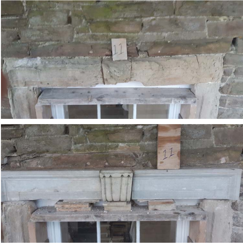
Figure 6.17: Window 11, Damer House, prior to repair (a); following repair (b). This was one of the more badly decayed windows.
