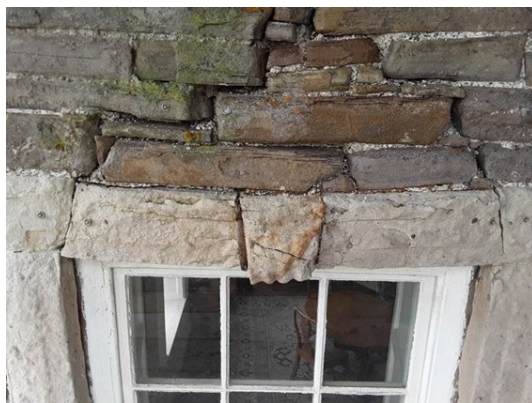
Figure 6.3: North façade, Damer House. Structural failure to window 1, with sagging of random rubble stone masonry.
