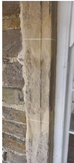
Figure 6.16: Repaired joint with lime repair mortar and simulated silica sand joint, Damer House. The repair mortar will harden and darken on exposure to the environment.
