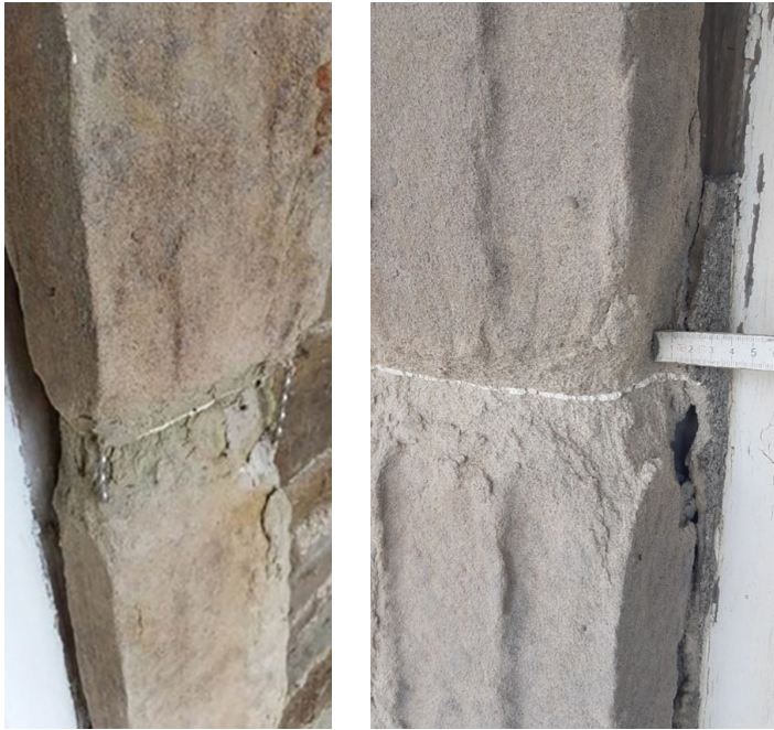
Figure 6.5: (a) Decayed joint between window jambs reinforced with stainless-steel helical bars, Damer House; (b) Erosion had produced significant gaps between the window jambs and the window sash boxes, Damer House.
