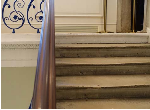
Figure 1.8a: The South Stair at the Queen's House. Detail of the top steps and the timber landing.
