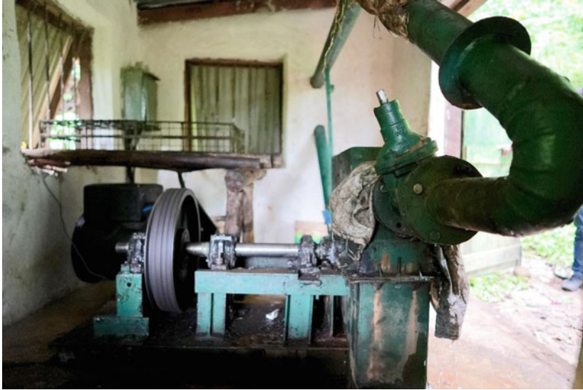
Fig. 10.5 The chipopoma power plant still relies on makeshift technology which is improved day on day
