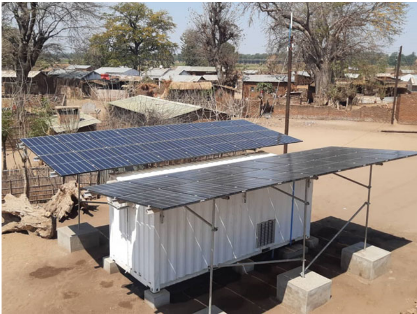
Fig. 5.6 12 kW solar micro-grid, Mthembanji, Malawi
