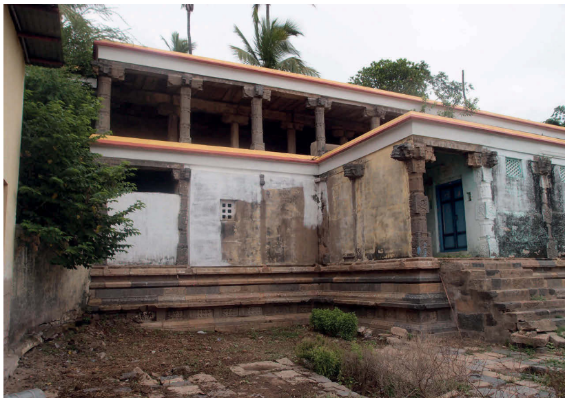
Fig. 6: View from the south-east. The library's pavilion with the new staircase and (to the left) the extension of the library in the gallery.
