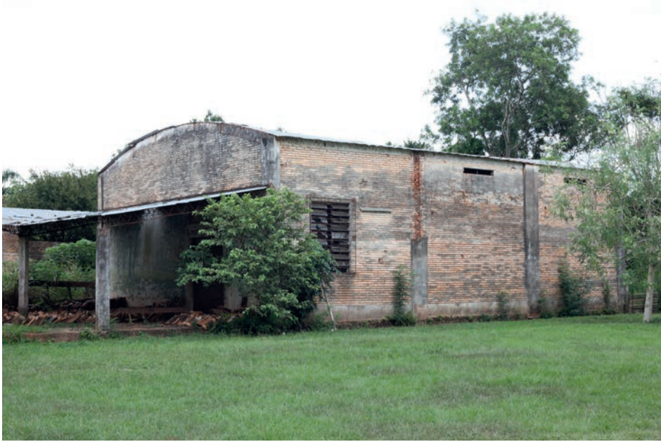
The buildings of the former Jopoi and the technical school are unfortunately falling into ruin
