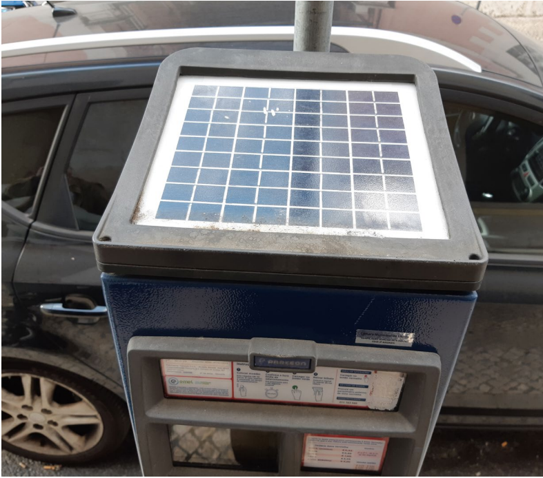
Figure 7.12 Solar PV integrated into parking meters in Lisbon. © The author
