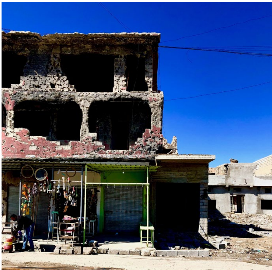
A partially destroyed residential/ commercial space 2019
