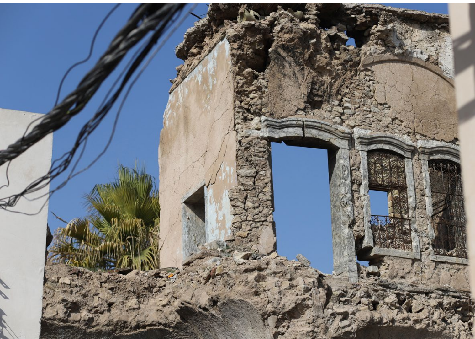
Partially destroyed building in the vicinity of the reconstruction site 2022
