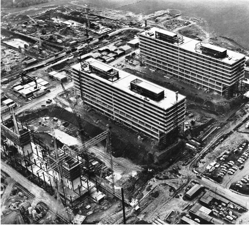
Fig. 11.2. Serial prefabrication of building elements in a field factory directly on the construction site of Ruhr University Bochum. Aerial view, status at the end of April 1965, H. Lohoff, Bochum (released by R. P. Münster, no. 0236/65).
