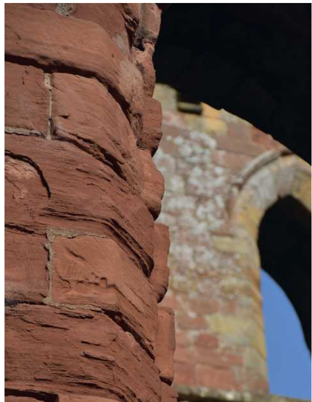
Figure 3.4: Weathered red sandstone of the St Bees formation at Lanercost Priory.
