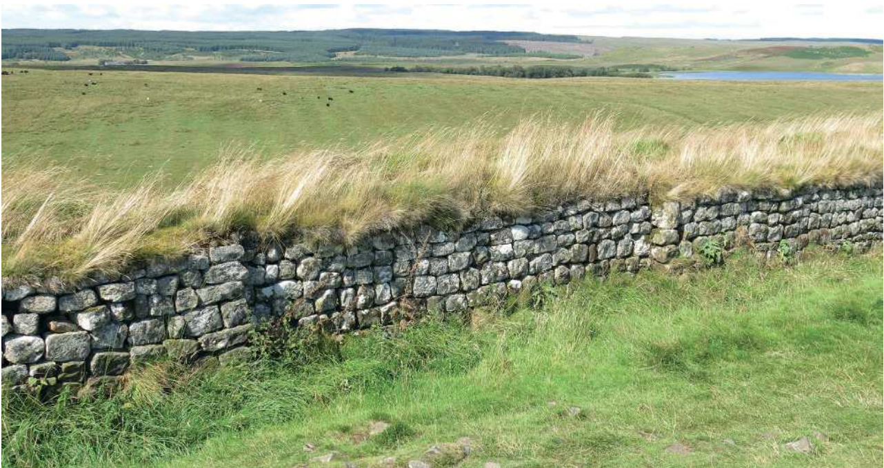
Figure 3.16: Projecting offsets visible on the south face of the Wall curtain in Wallmile 37, west of Housesteads fort. This location has two offsets in close proximity with a slightly narrower length of curtain between them.
