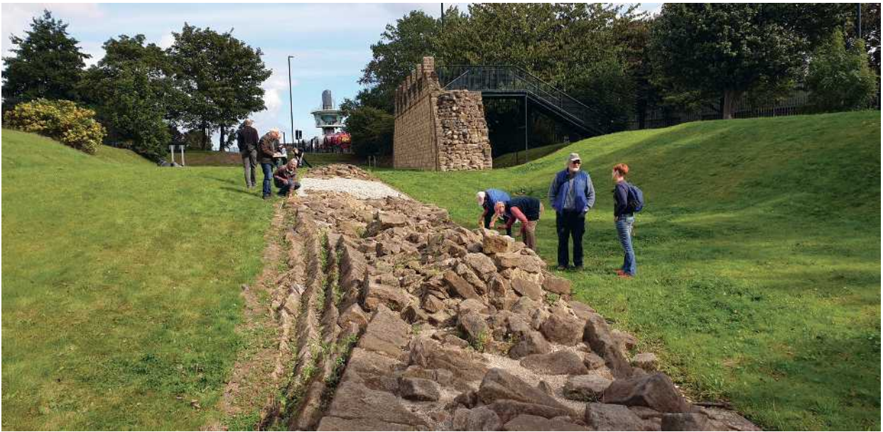
Figure 3.14: The consolidated length of Wall curtain at Buddle Street, Wallsend, which had multiple phases of collapse and reconstruction. Collapses introduced curves into the normally straight curtain, which were incorporated into rebuilds.
