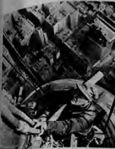
Television antenna is sixty-one feet above building. Wolff was assigned by Life to photograph installation of new antenna.
