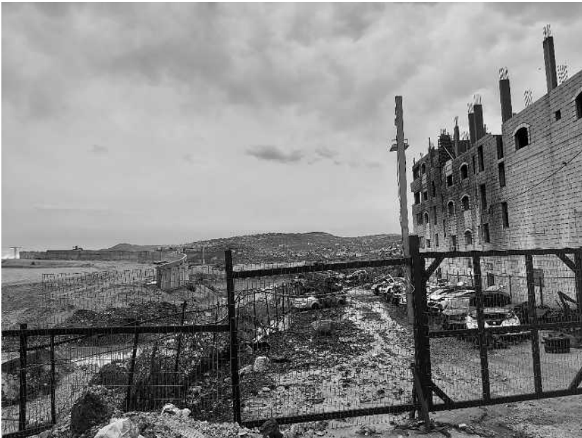
Figure 1: Segregated road being constructed for Israeli settlers near a Huwara apartment building subjected to a settler pogrom on February 26, 2023. Photo Credit: Zaha Hassan
