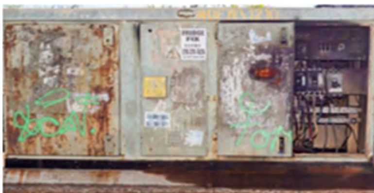
Figure 3. Status of transformers in Soweto (Author 2024).
