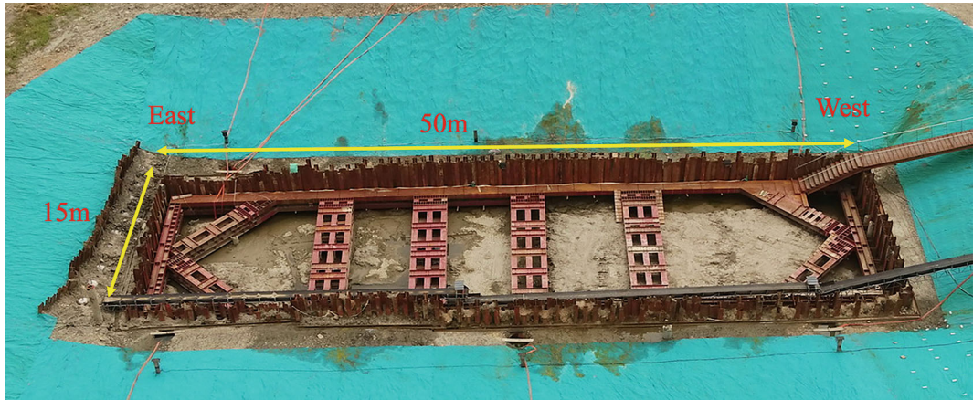
Fig. 10.4 Plan of sheet pile walls at the Jingtoushan site (Photo by G. P. Sun)
