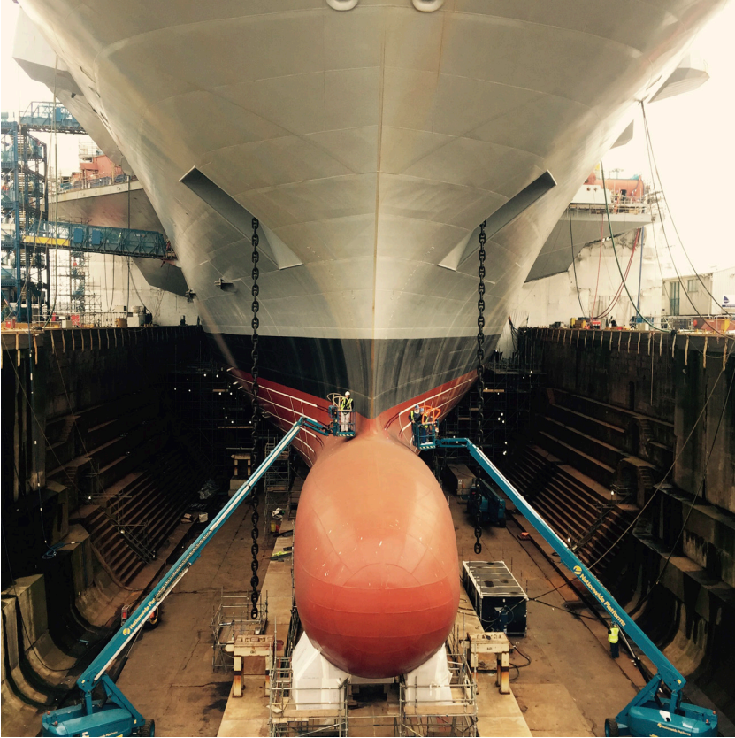
Figure 4.2: HMS Queen Elizabeth under construction. Photo copyright Chris Terrill. Used with permission.
