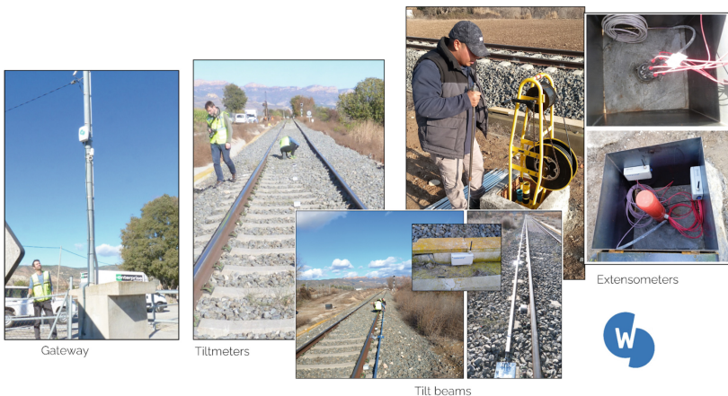
Fig. 9. IoT devices installed on the FGB railway track as a part of ICOS Railway Use Case
