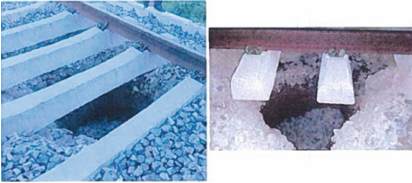
Fig. 8. Safety problem on the FGC rail track.
